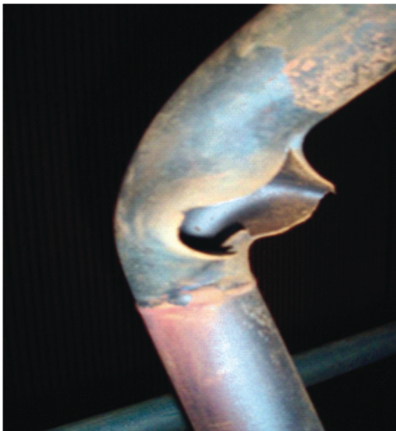
Figure 1. A rupture at the bend of a superheater tube
